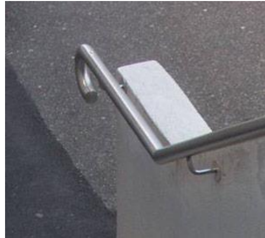
Figure 7.6: Compliant, rail extends beyond the stair
